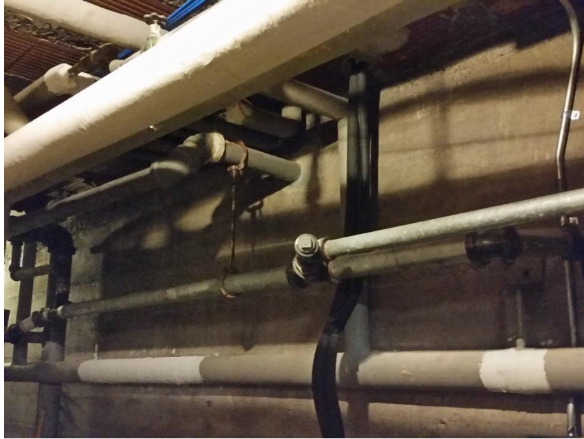
70+ Year Old Plumbing
