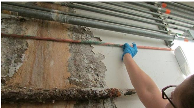
1. MCF-Moose Lake tunnel corrosion
