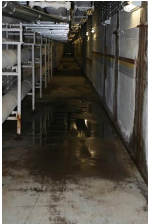
1. MCF-Moose Lake water running in due to roof and run-off from outside parking lot.
