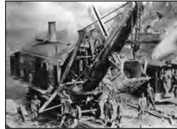
This steam-powered shovel was emblematic of the open pit mining on Minnesota's Mesabi Range during the first half of the 20th century.
