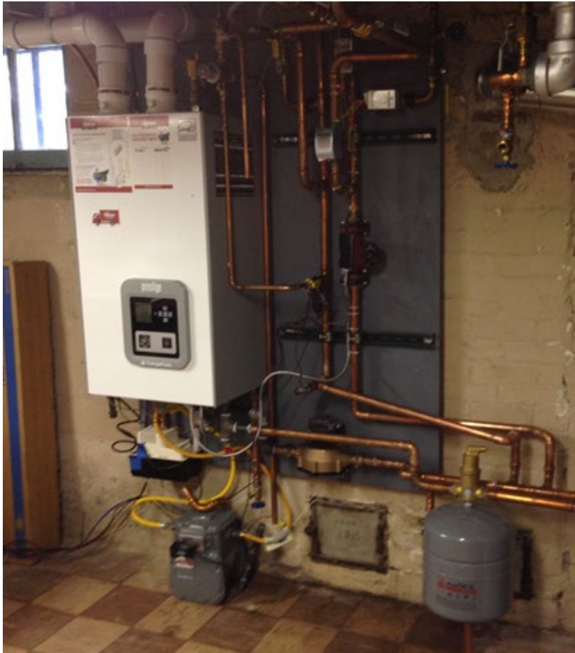
Figure 1: Existing Boiler at Site Exist_07
