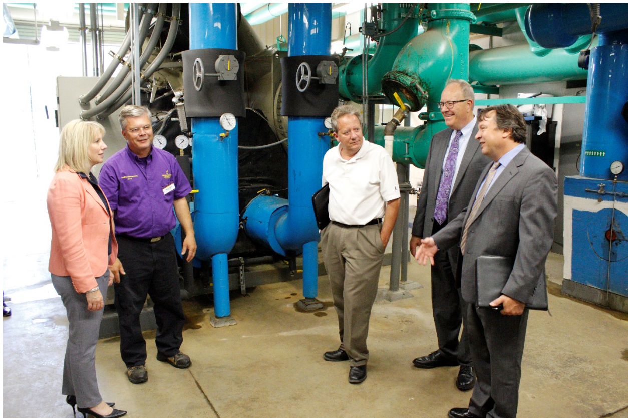
Commissioner Looman (left) got a first-hand look at several mechanical system upgrades at Minnesota State University-Mankato, with (left to right) MSU’s Steve Ardolf and Greg Borchert, Commerce’s Pete Berger, and MSU’s Paul Corcoran describing the successful energy-savings project.
