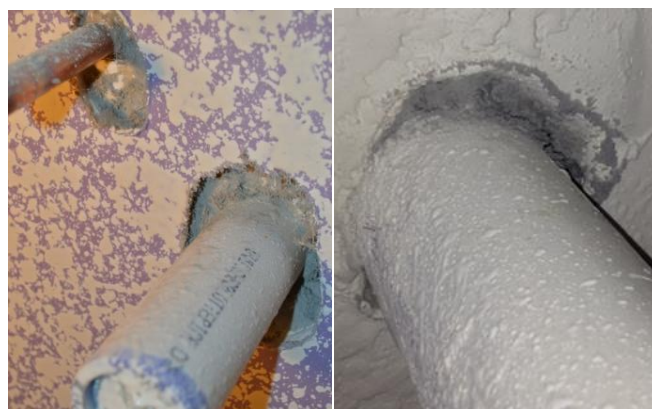
Figure E2. Visual images of sealed air leaks
