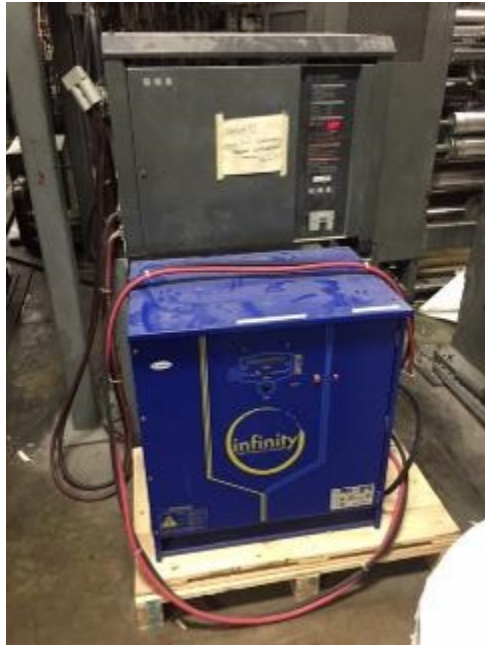
Figure 2. Battery charger station with existing and high frequency batteries being monitored (photo courtesy of Franklin Energy)
