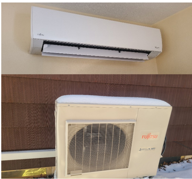
Ductless mini-split, one-to-one system
