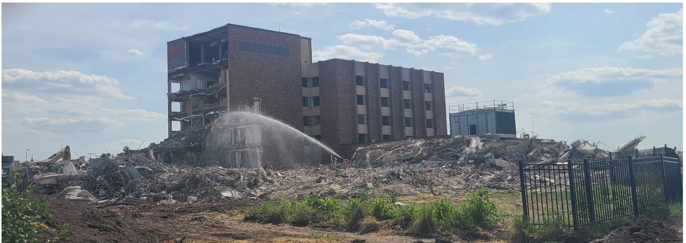
View from Como and @ Capitol Boulevard. Demolition of the former Bethesda Hospital began in late spring. Construction of the new behavioral health hospital will begin late summer or fall 2023.
