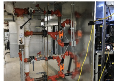
911 Call Center AHU New Castle County, DE
