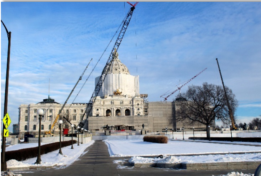
The Capitol Restoration Project is a massive interior and exterior repair, restoration and renovation initiative
