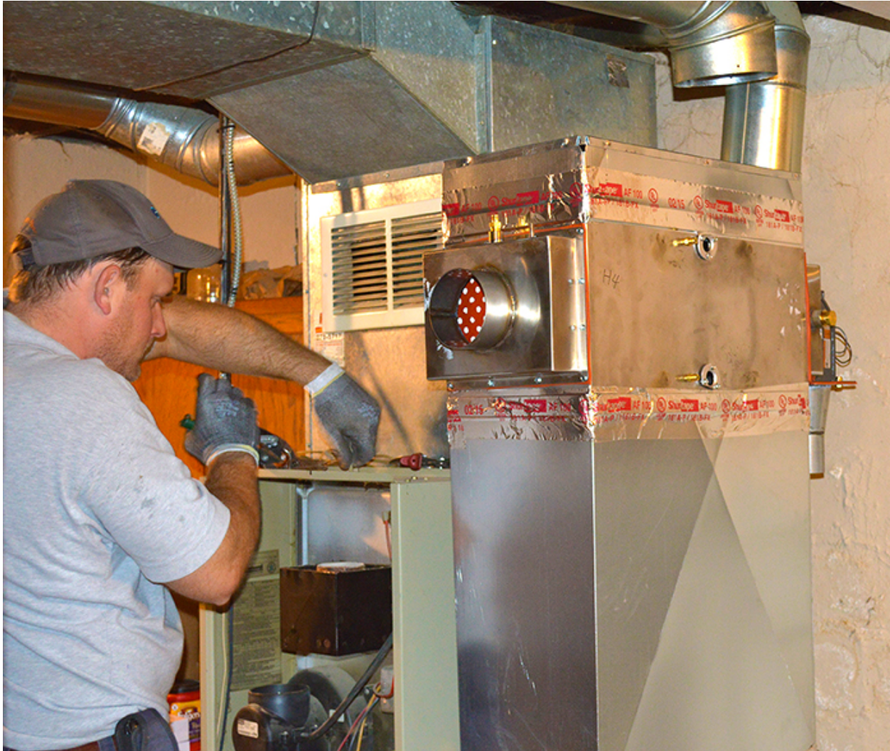
Figure 1. TMH device installed in one of the test sites
